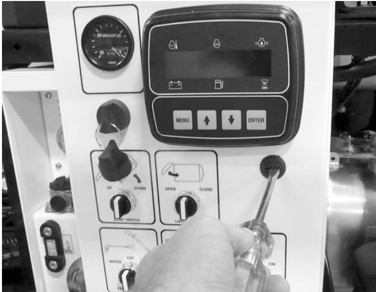
Figure 5-9. To access the fuse block, open the front of the curbside control panel.
