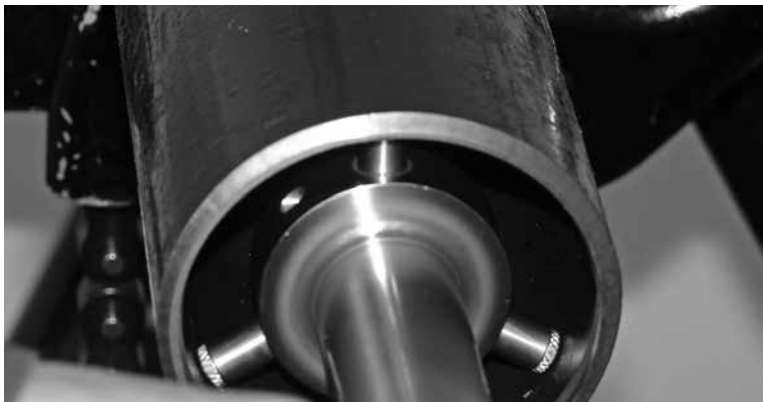
Figure 5-15. The mandrel legs should be close to the edge of the pipe.
