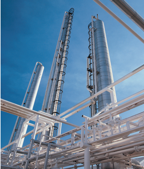
Figure 1 - Flange facing is an integral part of plant maintenance
