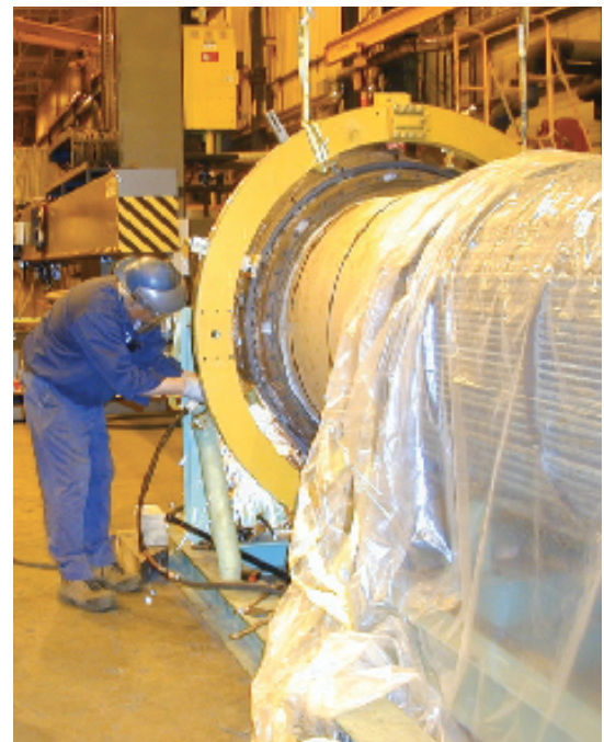
Fig. 6 — Split frame rotating ring cutting equipment sectioning welded shell, leaving a beveled, weld-ready finish.
